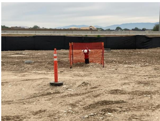
FIGURE 8-6B-3(a) HYDRANT FENCING
